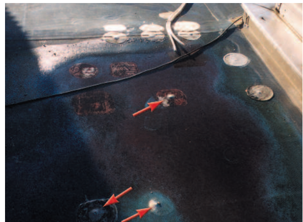
Figure 4 Arrows show where screw heads are pressing against the waterproofing membrane. A number of previous penetrations have been repaired. A pond of water is visible in the affected area
