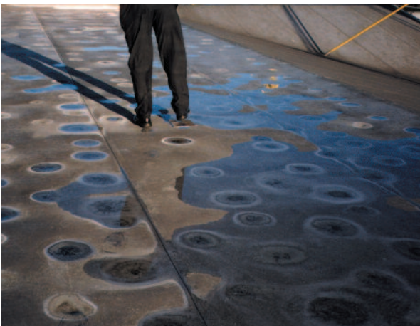
Figure 6 Patterns of deposits left by water pond evaporation can be seen. The polka dot pattern is due to individual ponds forming round single fixings which have been installed in such a way as to dig into the compressible rock mineral fibre insulation. They are not caused by collapse from foot traffic.
